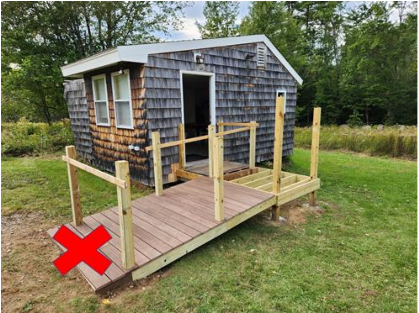
Was a multi-day effort so this was work in progress with no-access yet. Stairs on the left had to be used in the meantime.
